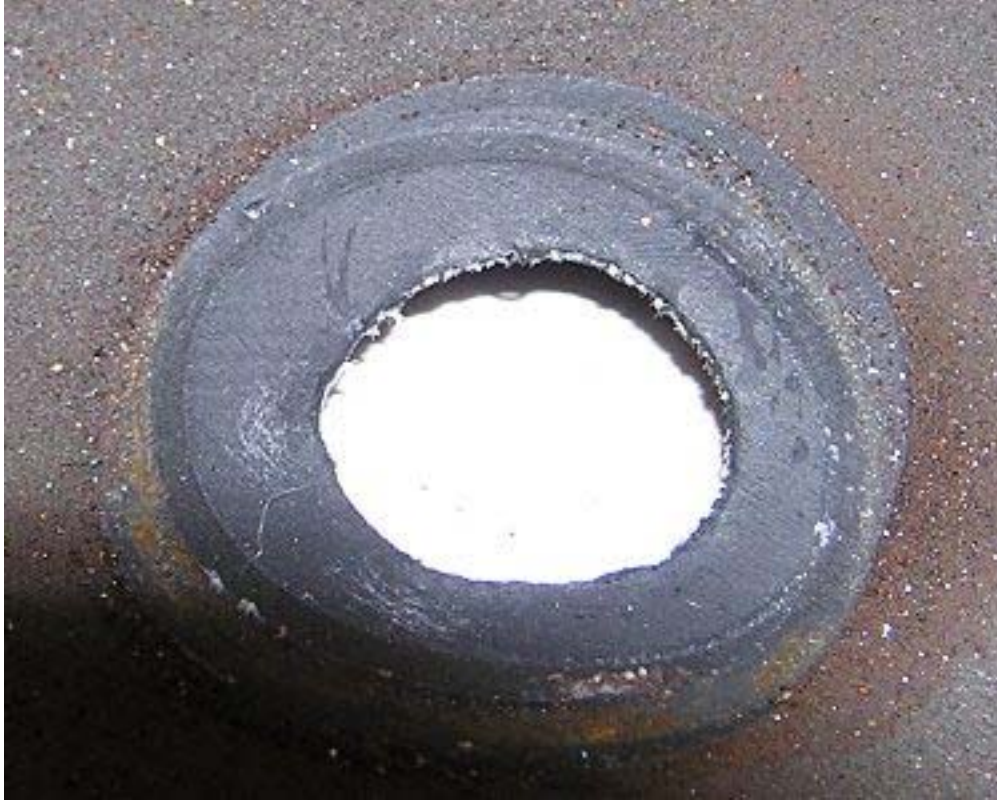
Figure 5: Removed Debris on Seal Between Diaphragm Bottom and Control Linkage
